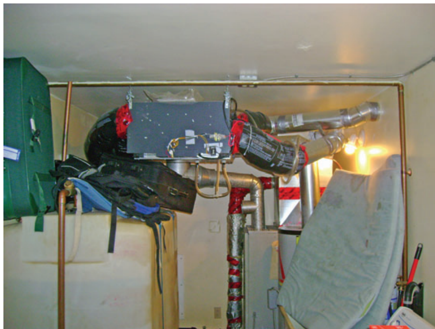
Fig. 3 Photograph of a Venmar Constructo 1.0 heat recovery ventilator installed in the furnace room of a study house
